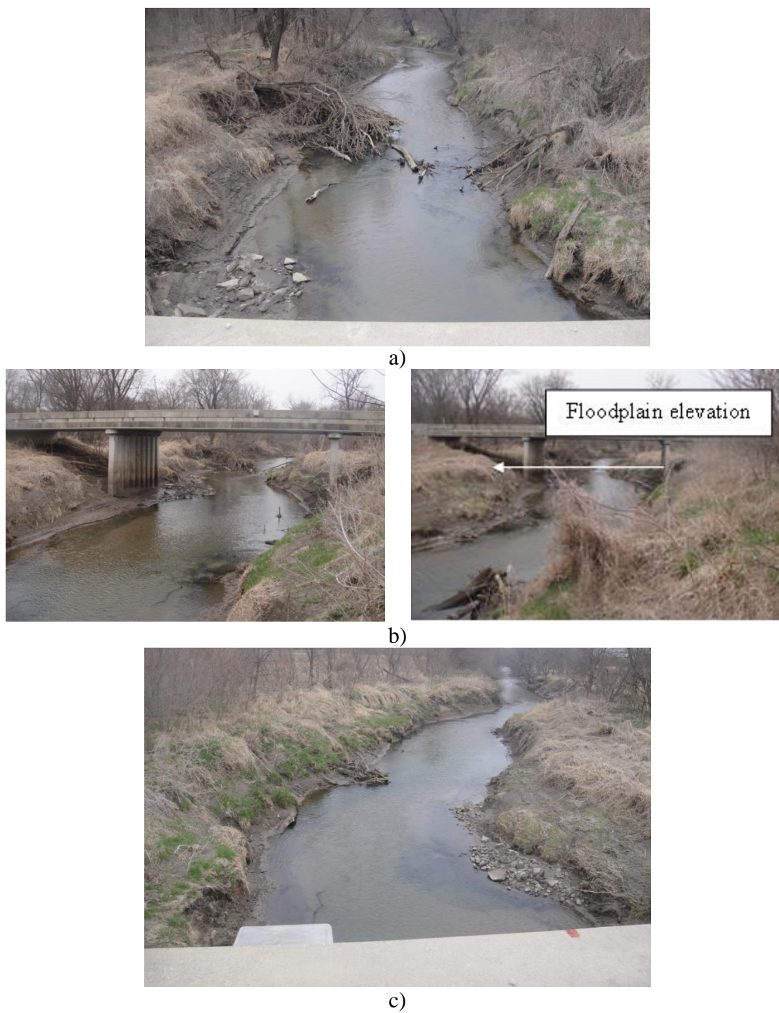
Figure III.2 Site conditions at Clear Creek on April 4, 2011: a) Upstream view; b) Bridge view c) Downstream view
